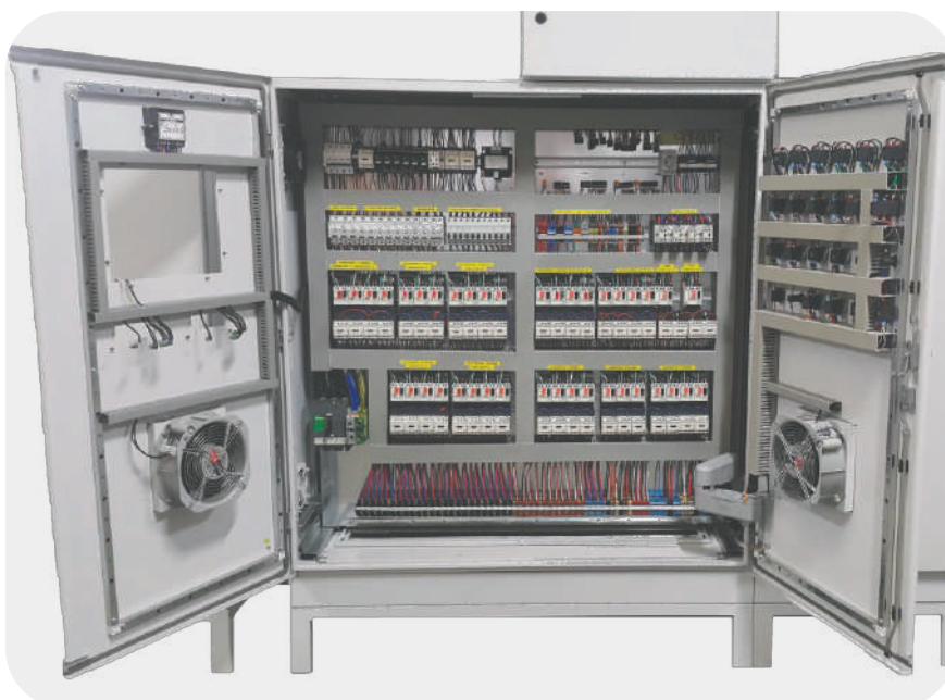
Figure 23: Inside View of Electrical Panel
